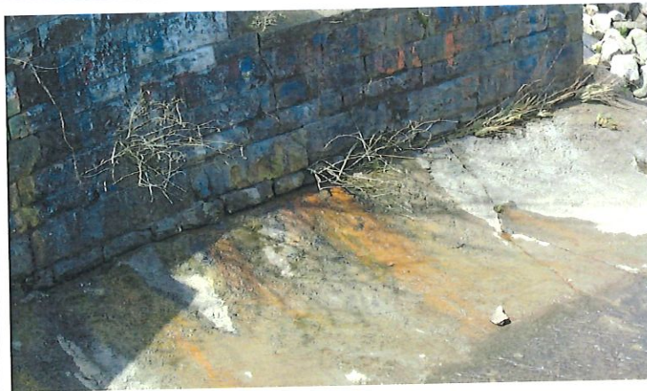
11. Photograph from April 18, 2018; iron staining is indicative of seepage.
