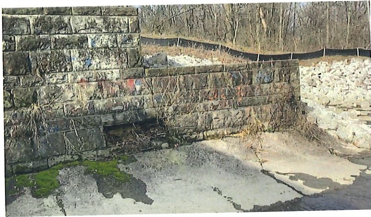
10. Left sidewall at the principal spillway outlet; seepage has been reduced compared to previous observations (see Photograph No. 11)
