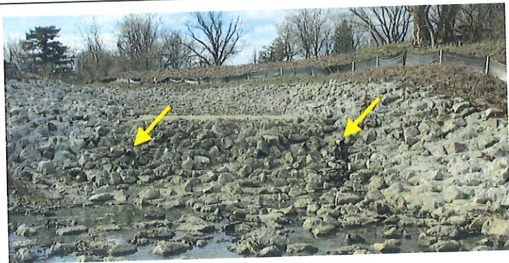
13. Emergency spillway outlet; arrows point to the underdrain outlets; left (referenced looking downstream) had trickle flow, and the right was dry.
