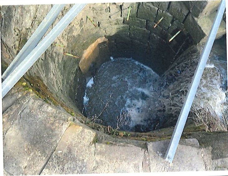
7. Interior of the principal spillway riser; no leakage noted and free of obstructions.
