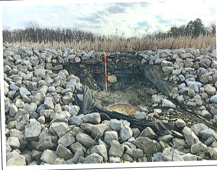
15. Close up an eroded area.
