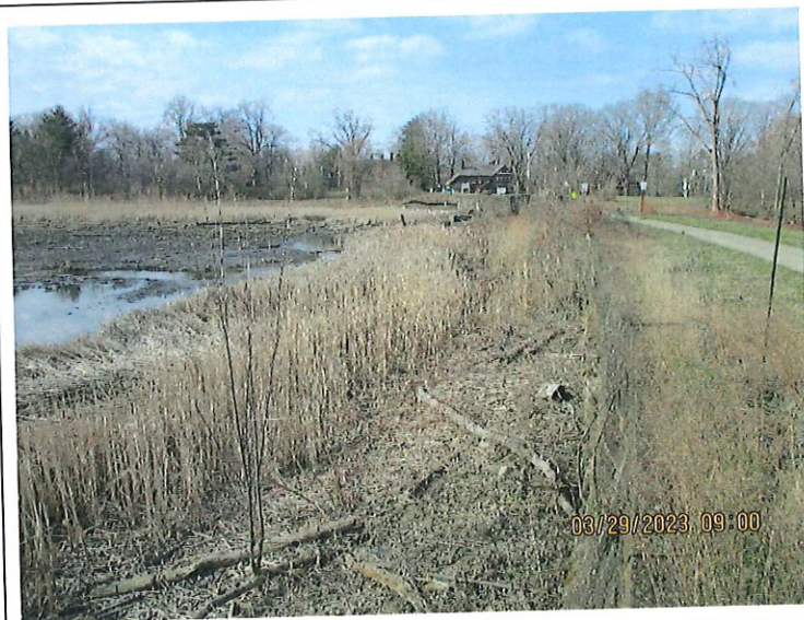
3. Upstream slope looking toward the principal spillway. Notice the tall brush and saplings along the masonry wall (former shoreline).
