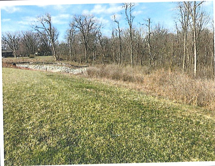
2. Grassed portion of the right downstream slope; notice the vegetation encroaching upon the toe area.
