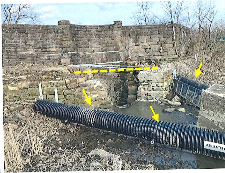
6. Principal spillway inlet area. The dotted line indicates the former normal pool level. The arrows point to the trashrack/debris collection system to keep the low-flow inlet clear.
