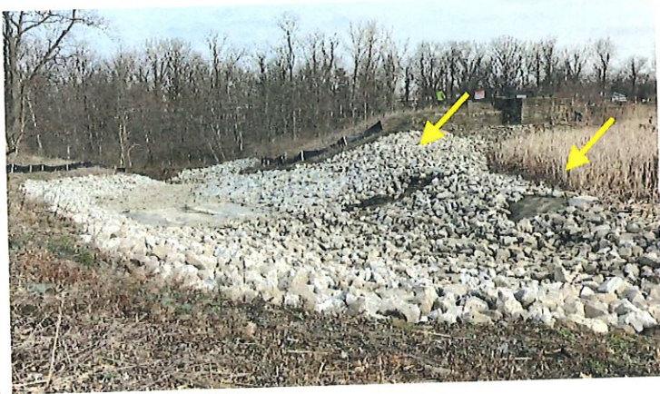
14. Emergency spillway channel inlet area; arrows point to eroded areas.
