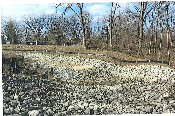
12. Overview of the area where the principal spillway and emergency spillway combine to flow into the receiving stream.
