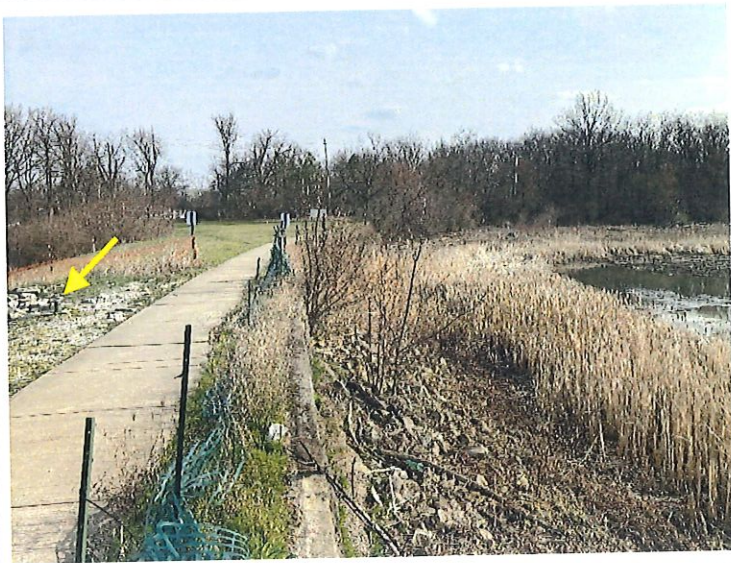
4. Upstream slope looking toward the right end. Notice the tall brush and saplings along the masonry wall (former shoreline). The arrow points to a piezometer.
