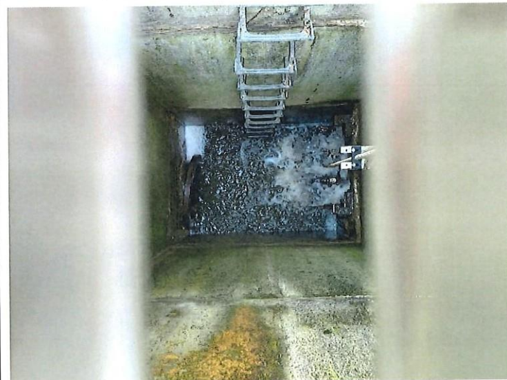
12. Interior of the well; no leakage or obstructions; no noticeable defects with the operator.
