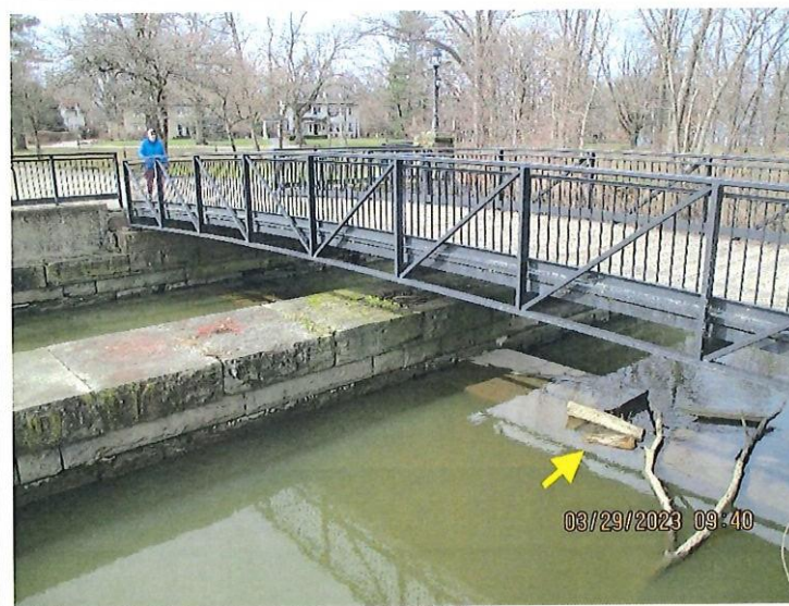
3. Right side of the spillway under the bridge. The arrow points to a flashboard, but its purpose is unclear because the downstream wall is the control.
