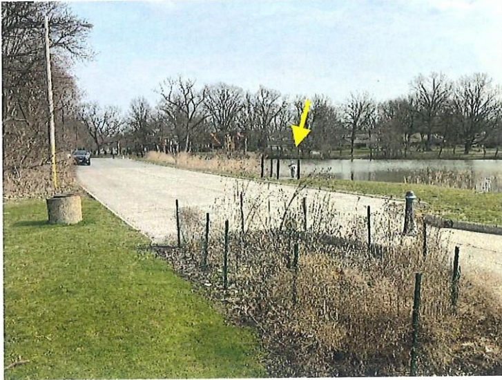
10. Overview of the crest viewed from the right side of the principal spillway. The arrow points to the lake drain well and operator.
