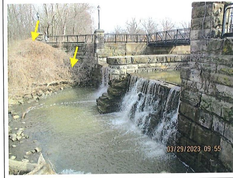
6. Overview of the spillway outlet area. Notice the vegetation by the right sidewall (arrows). The masonry structure was deteriorated and the undermining at the outlet is unknown.
