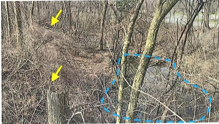
13. Downstream slope viewed from right end of dam; the wet area is circled; arrows point to the downstream slope.
