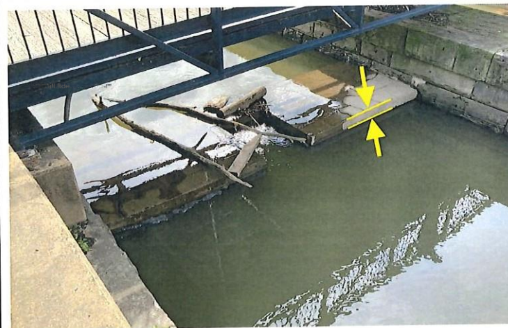
18. Right side of spillway; notice that the stop logs are in place, create about 0.3-foot water surface elevation difference between the pool and the downstream overflow wall.
