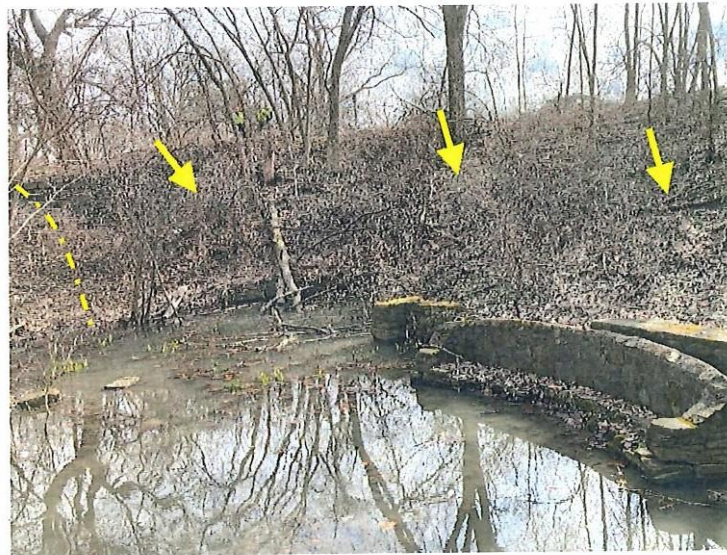
14. Downstream slope viewed from toe looking toward the right end of dam; arrows point to the downstream slope.
