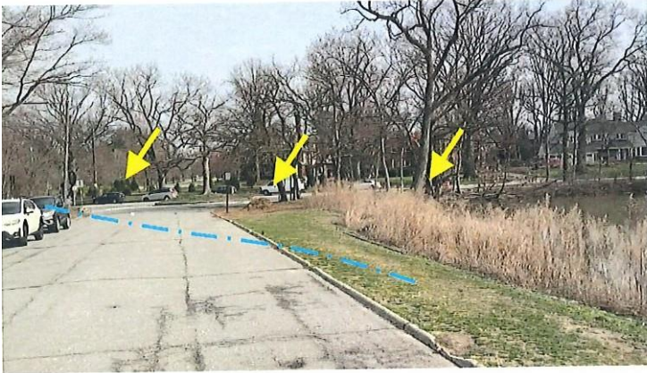
16. Overview of the right end of dam; arrows point to the low area/emergency spillway.
