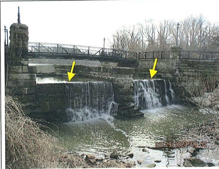
4. Overview of the spillway outlet area. The arrows point to the downstream wall that controls flow.
