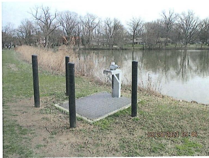
11. Lake drain well and operator.
