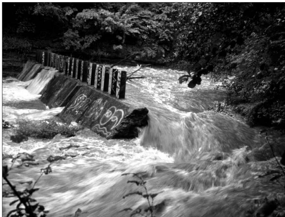
Figure 7-4 Erosion around the end of the trash rack upstream from Martin Luther King, Jr., Boulevard is one result of high flows in Doan Brook. Photograph by L. C. Gooch
